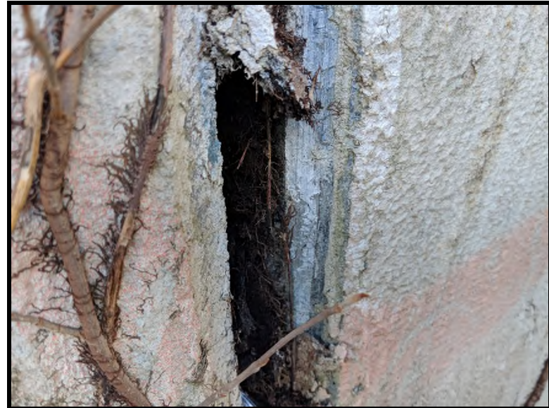
6 The expansion joint material and textured material tested negative for asbestos.
