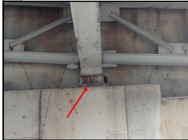
4 The gray metal support plate tested positive for lead-based paint (1.70 mg/cm 2 ).
