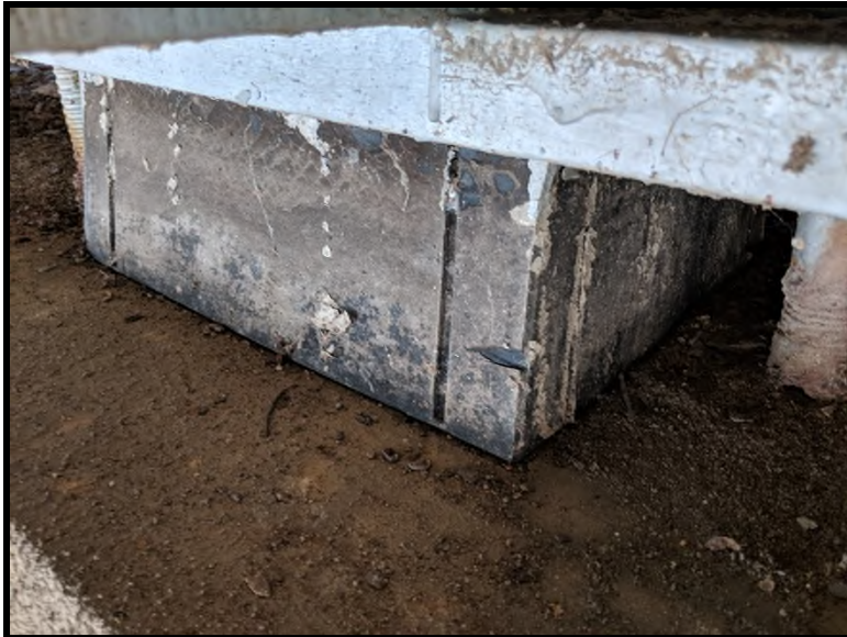
5 The rubber blocks located on the east side of the bridge were considered non-suspect material.
